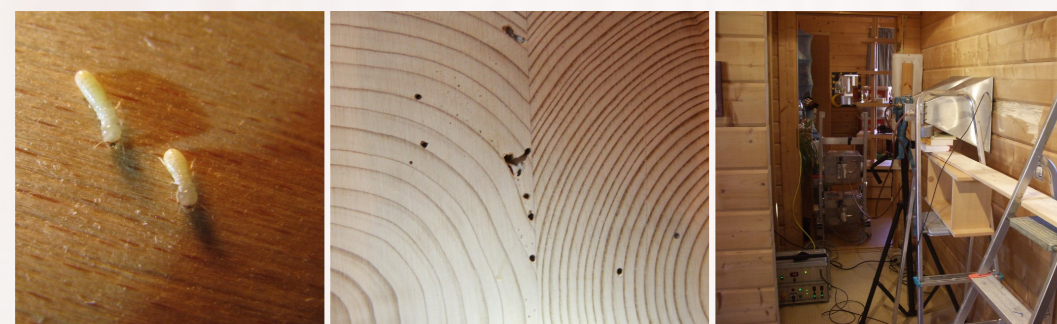
Figure: 1-3 Drywood termites Kalotermitidae in a wooden wall (2008 Kirchroth)
